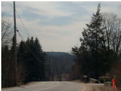
Picture Limited visibility of extremely sharp turn on Pudding Hill Rd makes a dangerous situation
