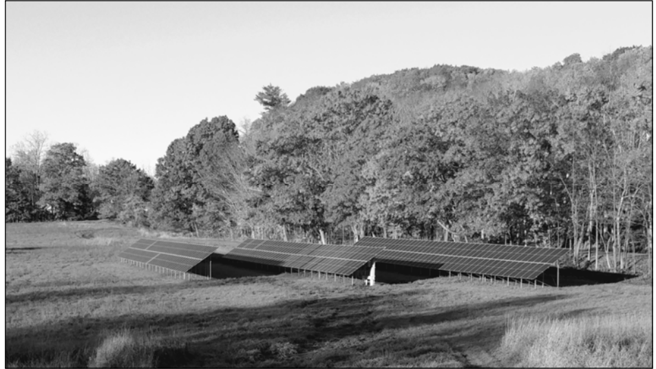
Madbury's town solar array next to the Safety Complex on Knox Marsh Road.
