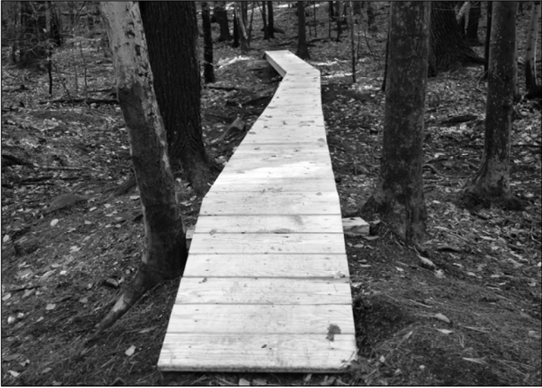
The replacement boardwalk on Hicks Hill courtesy of the Seacoast Chapter of the NE Mountain Biking Association, with support from the Conservation Commission.
